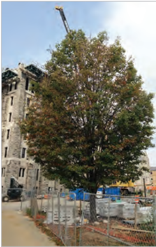
Construction activities compact the critical root zone. Photo: Eric Wiseman, Virginia Tech
