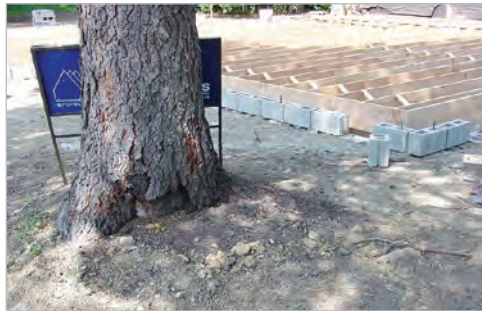
Foundation is very close to this maturing tree. Photo: Andrew Koester, International Society of Arboriculture, Bugwood.org
